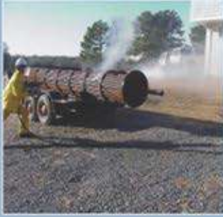
External Tube Bundle Cleaning
